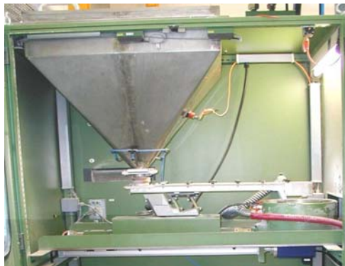
Dosing device, fully air-conditioned
